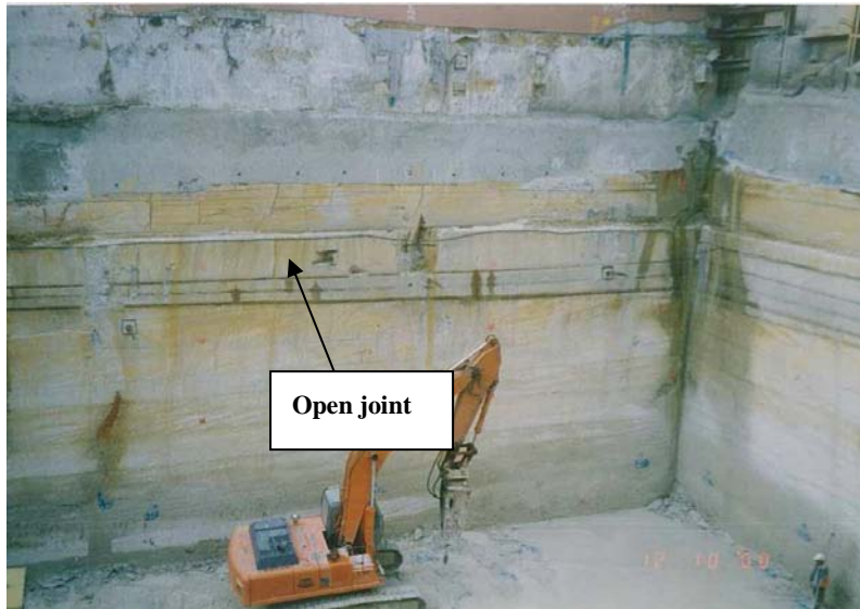
Figure 8: General view of UTS face at end of basement excavation showing location of open joint and subhorizontal laminite bedding seams.
