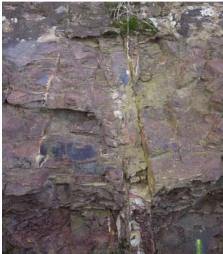
Figure 9a: Through going joints in road cutting at Bald Hill, just north of Stanwell Park.
