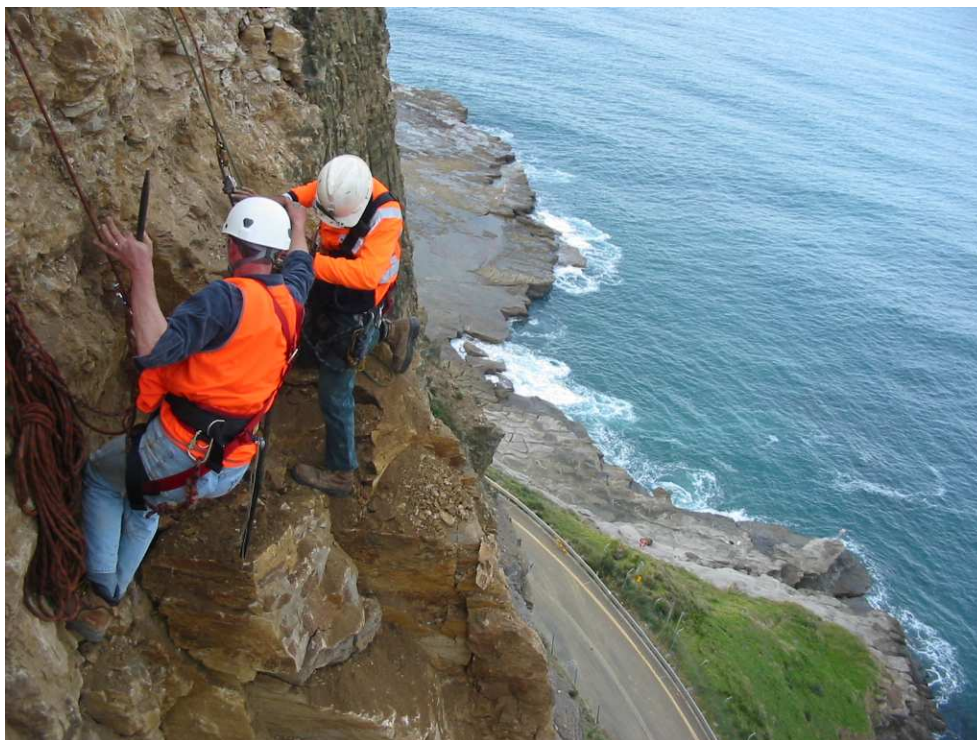
Figure 5: Engineering Geologists supervising scaling works in GD5. Note rope and equipment set up and Lawrence Hargrave Drive about 40 m below.
