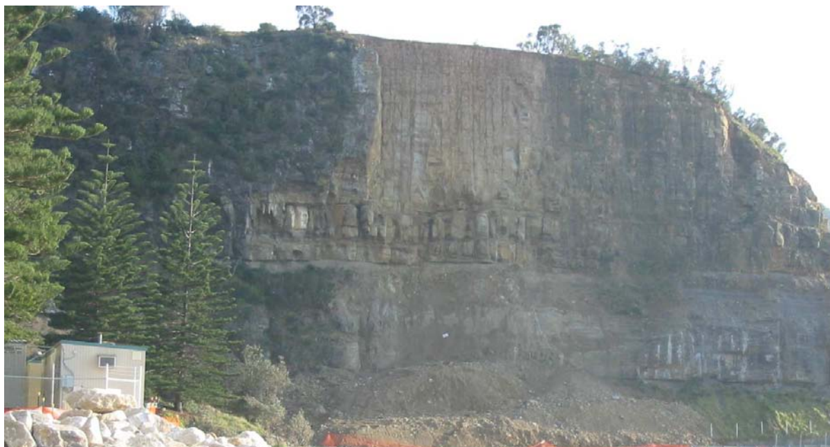
Figure 4: View of GD5 showing cliffs in Scarborough Sandstone following blasting undertaken as part of the geotechnical remediation. The cliffs were subsequently scaled and additional support provided by rock anchors and rock fall mesh. All work, including drilling for rock anchors, was carried out using rope access methods.
