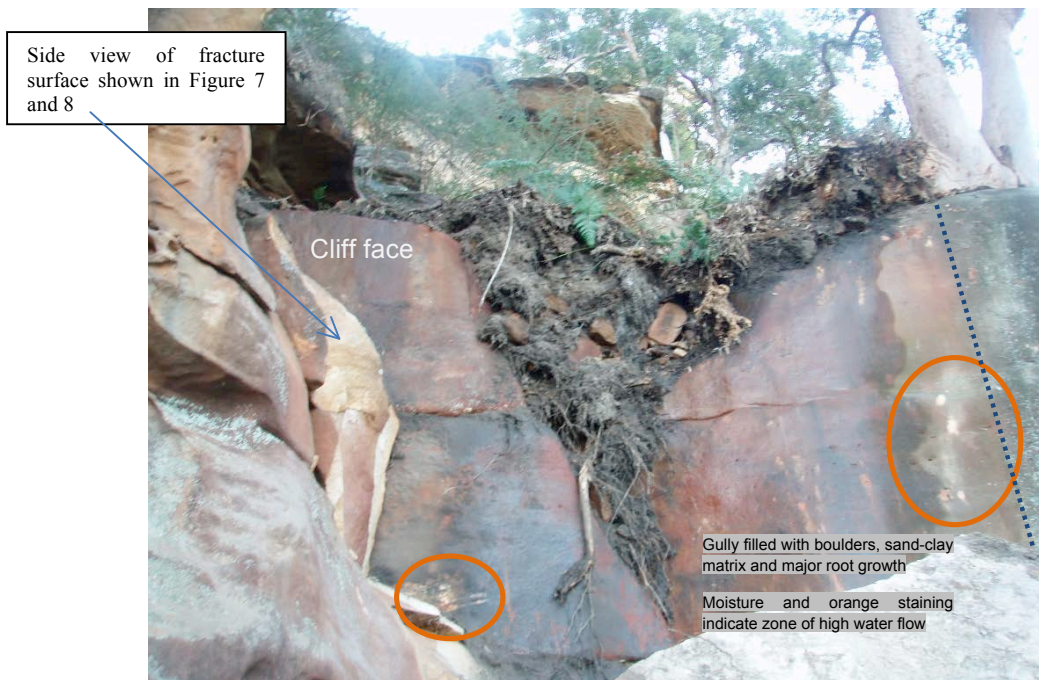
Figure 9: Large gully within rear wall of cliff, exposing one surface of the Joint, J2 (Figure 4).
